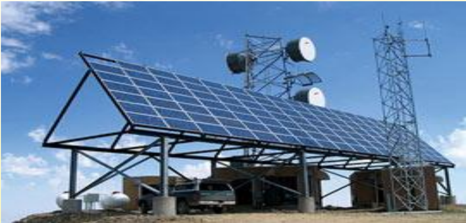
[Solar Operated Telecom Tower ]
