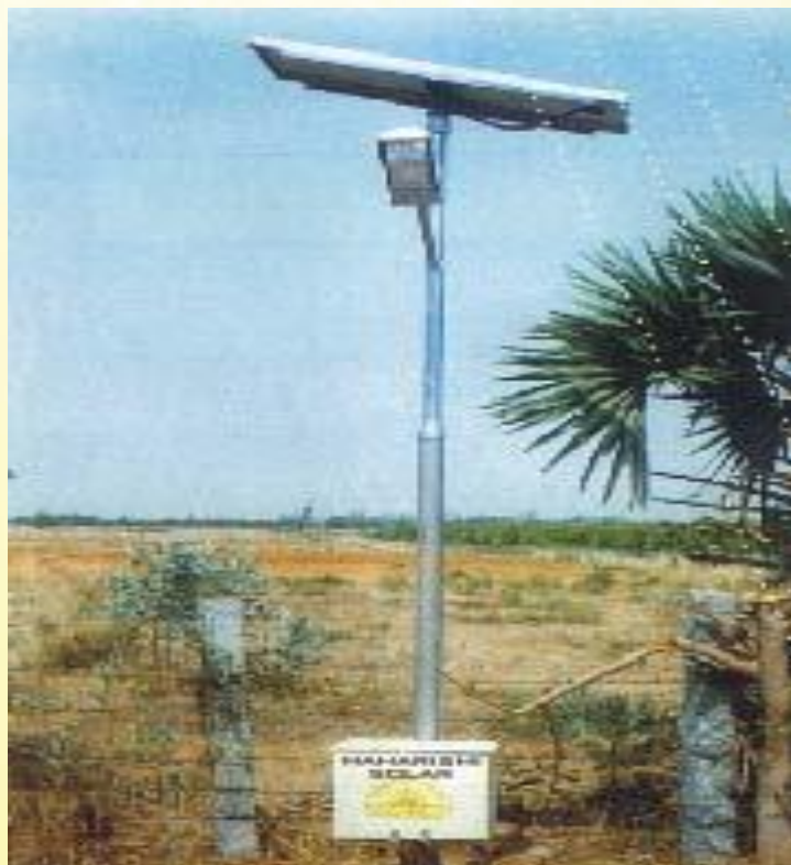
[Solar Street Light]
